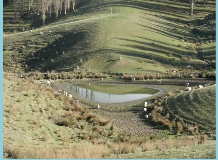
An old dam originally built with a horse scoop, but topped up by bulldozer, failing in the 2009 drought.
